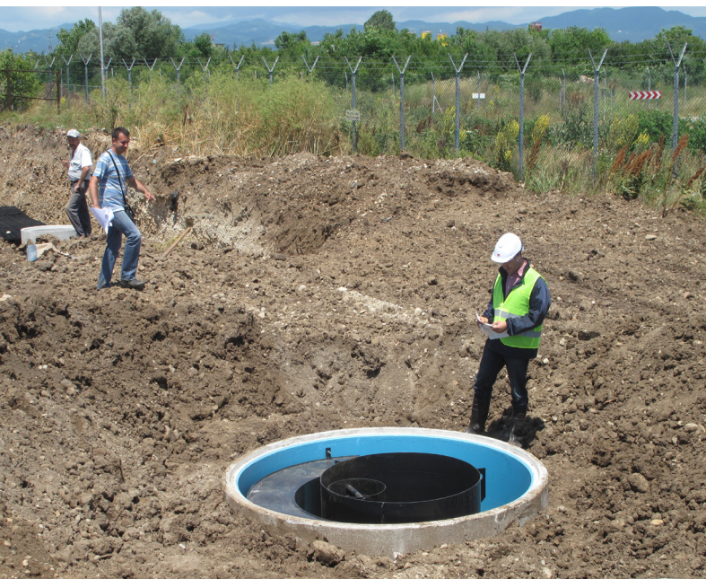
ACO Design and Service team supported each step of the design and installation
